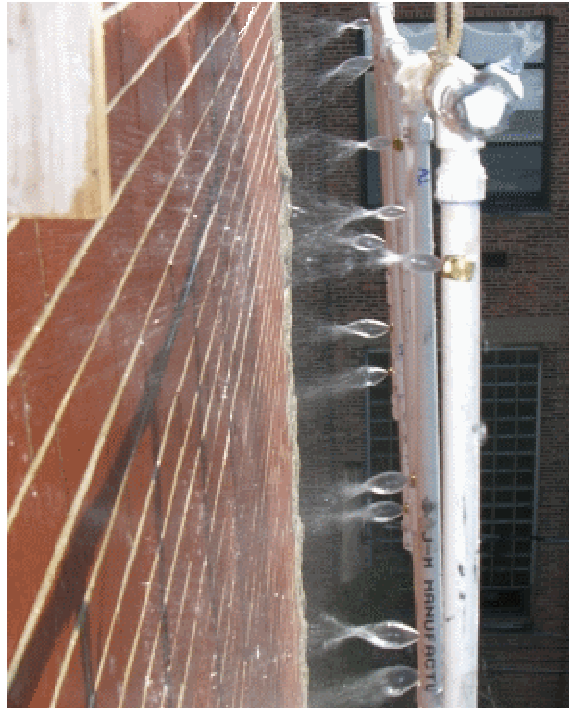
Spray rack on exterior face of masonry wall
